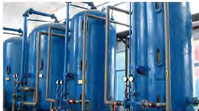
Boiler Softening Water
